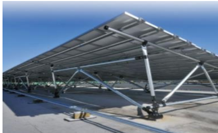
Solar Panel Structural Support
