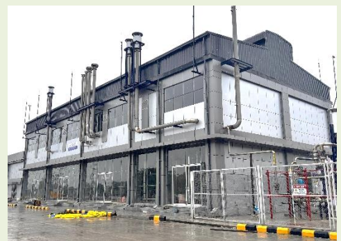
Green Hydrogen Electrolyser at Vijayanagar
