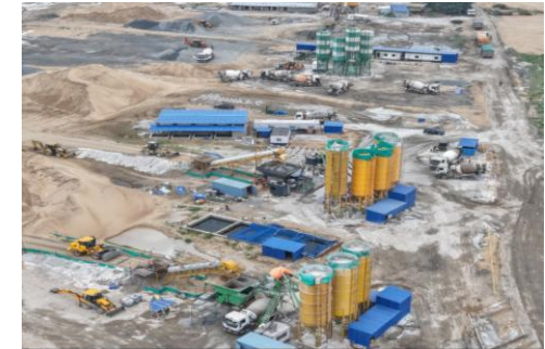
Batching Plants at Jagatsinghpur, Odisha
