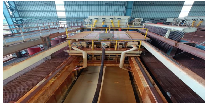
2 nd Filter Press at BPSL
