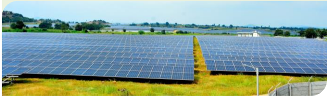
Solar Power at Vijayanagar
