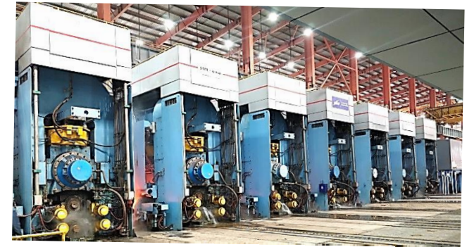
Finishing Mill in HSM at JVML-Vijayanagar
