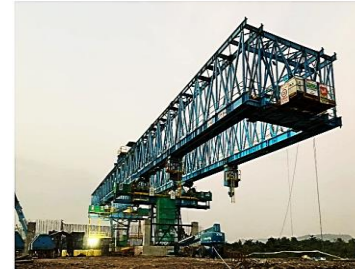
Launching Gantry (to lift and support bridge segments or girders) (S550MC – HR)
