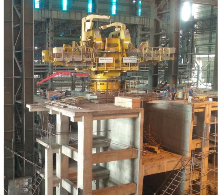
Ladle Turret & Casting Platform at SMS-2, BPSL Phase-II
