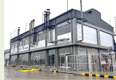
Green Hydrogen Electrolyser at Vijayanagar
