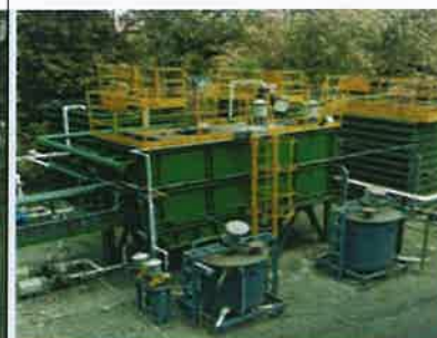
Rapid Clarifier System
