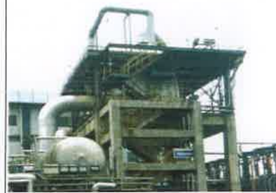
Multiple Effective Evaporator for ZLD plant
