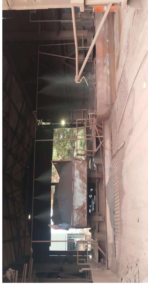
Sprinklers for Dust Suppression at truck unloading station
